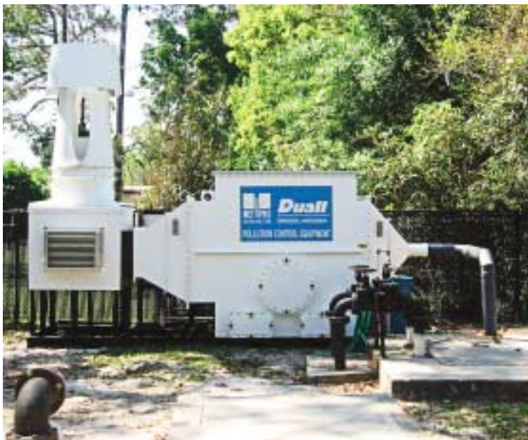
Duall installed a 400 cfm AroBIOS bioscrubber designed to treat up to 120 ppmv of hydrogen sulfide at JEA's lift station.
